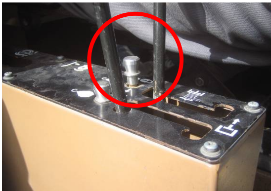
Free fall main and auxiliary hoist controls are not positively interlocked or fail safe.
